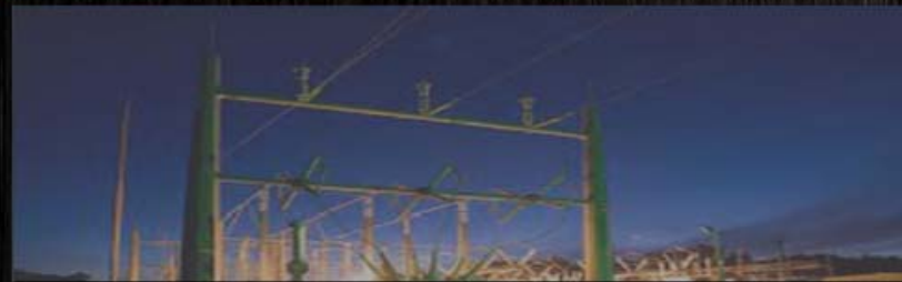
Our E-Houses lighting up a Leading Distribution Company
